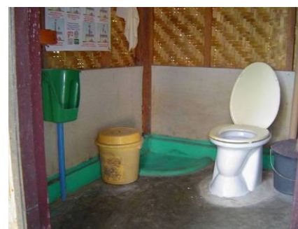
Figure 9: Inside a UDDT (source: DILG-GTZ Program)
