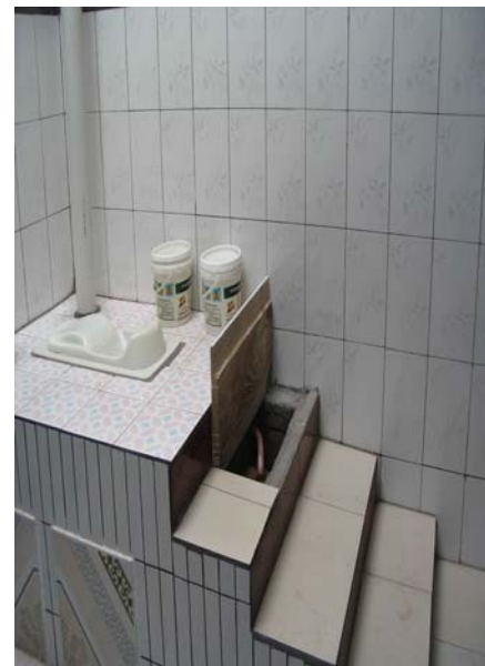
Figure 3: Access to the urine pipe and urine storage tank (source: Plan China)
